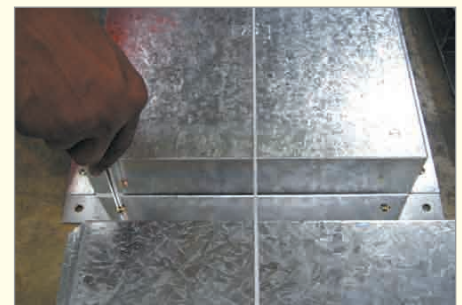
4. The side plates are to be removed and the trunkings are to be fastened with the junction boxes using self tapping screws.
