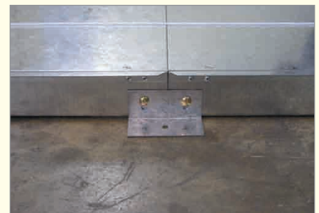
3. Join two trunking bases using fixing brackets and then fasten it to the slab. Ensure trunking alignments are as per guideline.
